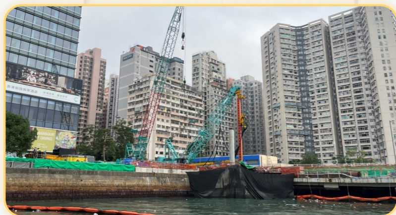
近糖水道碼頭連接橋的海上樁柱工程正進行中 Marine piling works near Tong Shui Road Pier Access Bridge in progress
